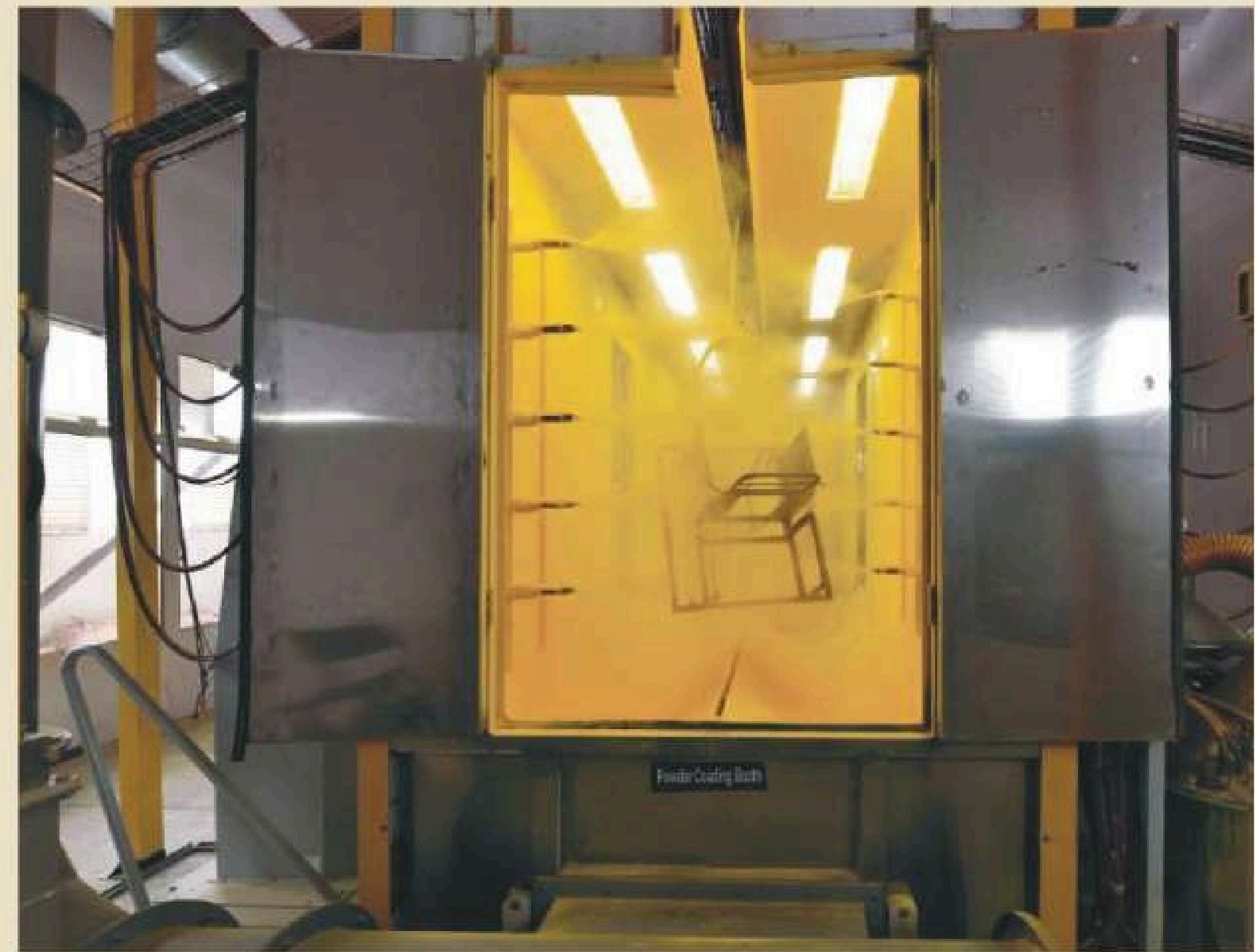
Powder coating booth at work center-6.
